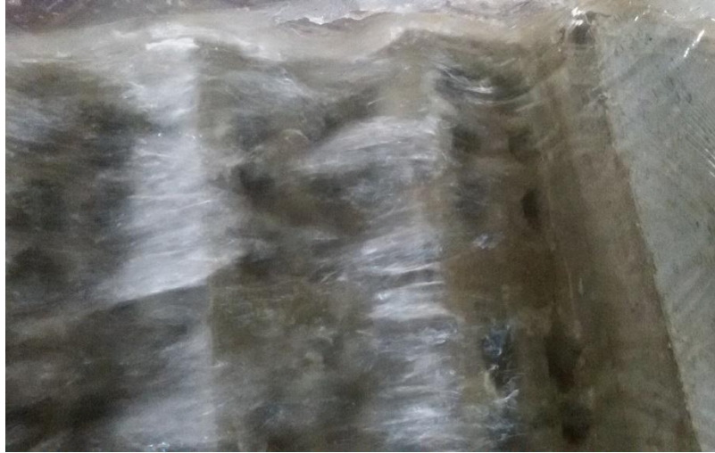
Figure 7. Stepped spillway provided with cavitation.
