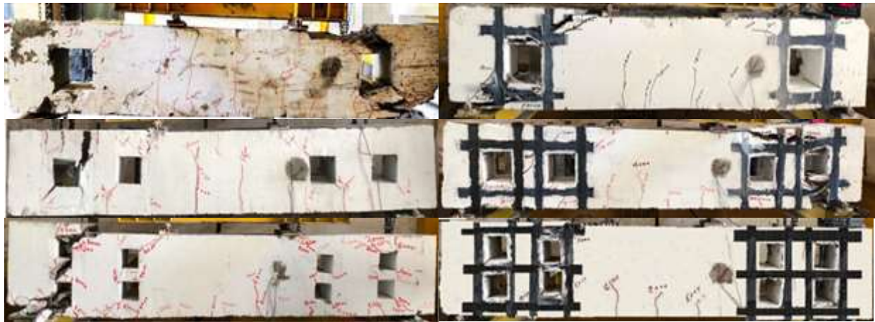
Figure 11. crack patterns of beams with opening.
