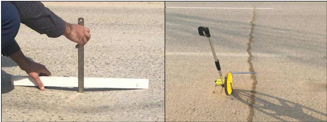
Figure 1. Pavement distresses measurements.
