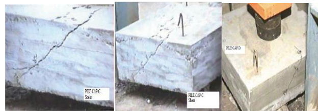
Figure 6. Four-Pile Cap Load Position and Shear Failure (Ahmed et al., 2009)
