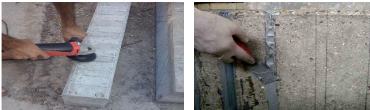
Figure 4. Roughing concrete surface and applying epoxy at CFRP strips location of a typical tested beam.
