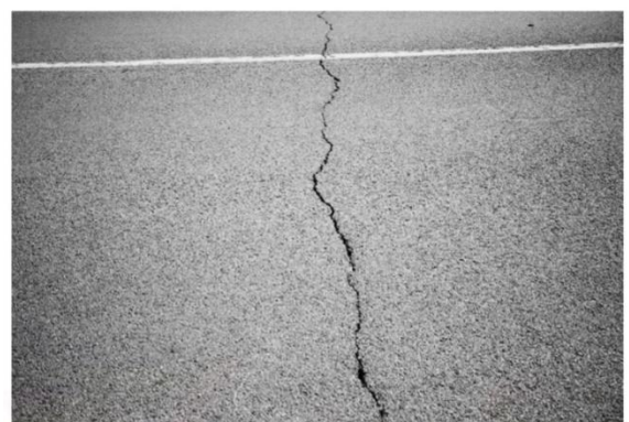
Figure 4. Rutting : longitudinal depression caused by the passage of vehicles in the wheel tracks path of a flexible pavement.
