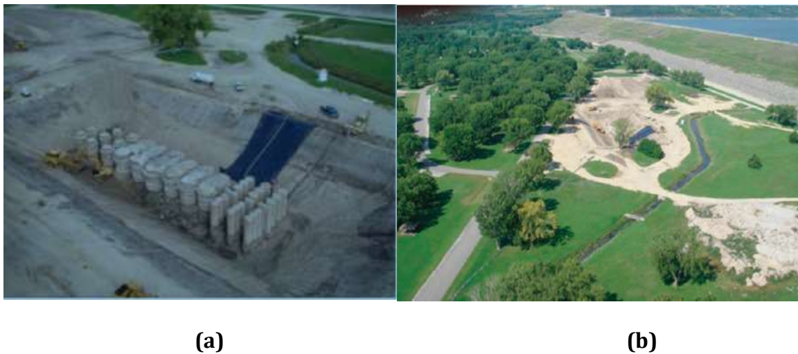
Figure 7. (a) View of Tuttle Creek Dam (b) Downstream of the Dam with Jet Grout (Stark et al., 2009).
