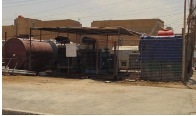
Generators smoke, spilled fuel and appearance
