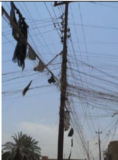
Crossed over electric wires
