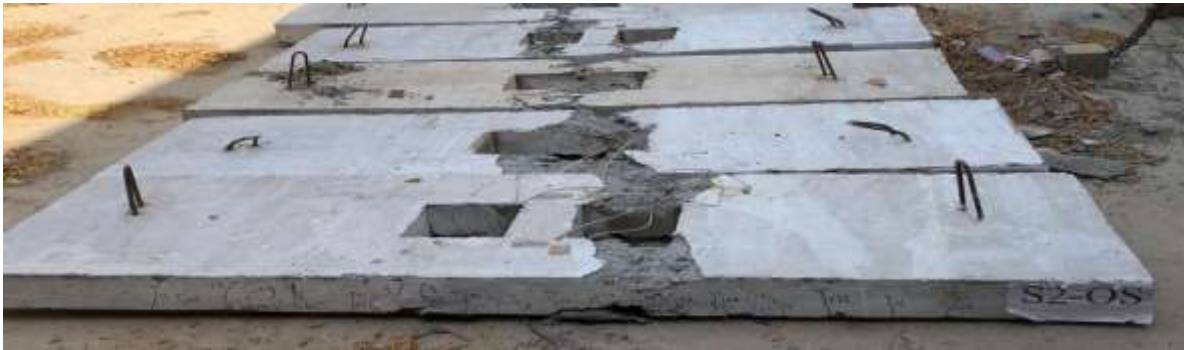
Figure 5. Slabs with GFRP bars after failure.
