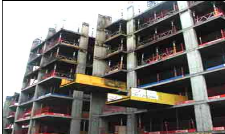
Figure (1): The concrete frame of a ten-storey building that was fire-damaged during construction, [Georgali and Tsakiridis, 2005].
