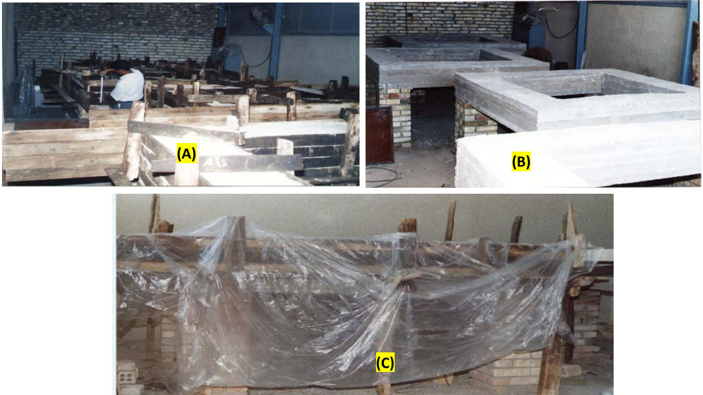
Figure (4): (A) The wood formwork of the rigid beams; (B) The rigid beams after lifting of the wood formwork; (C) Curing of Rigid beam with the wetted hessian and polythene sheets.
