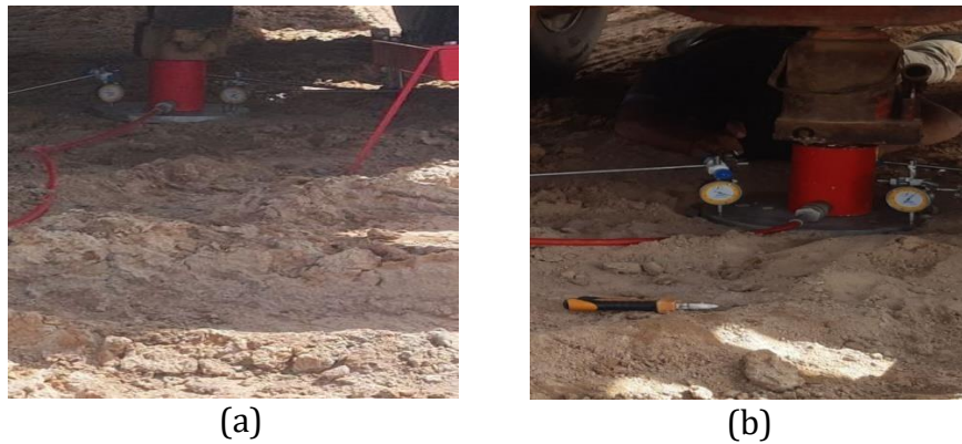
Figure 2. Plate bearing Test: a) Loading system, b) loading steel plate with three settlements.
