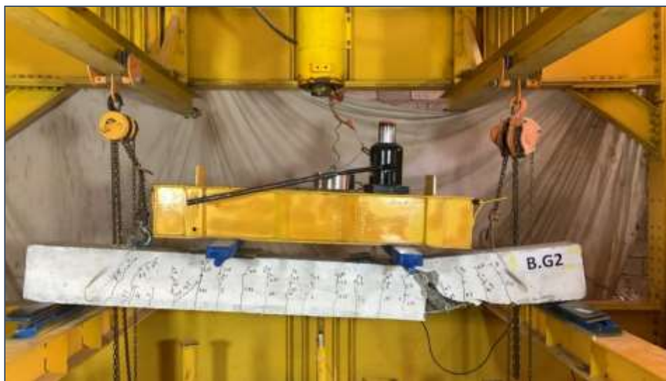
Figure 8. The failure pattern of B.G2 beam.
