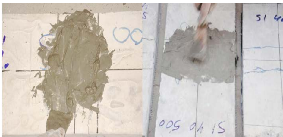
Figure 3: Repair of damaged and spalled areas of concrete with mortar (1 cement + 1 sand) at top and bottom surfaces.
