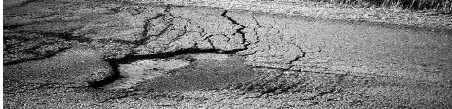
Fig (11) Slippage Crack at AL-Huriya City
