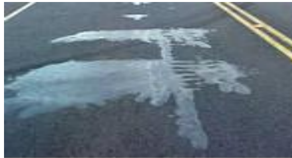
Fig (3) Bleeding at Al-Hamra'a City
