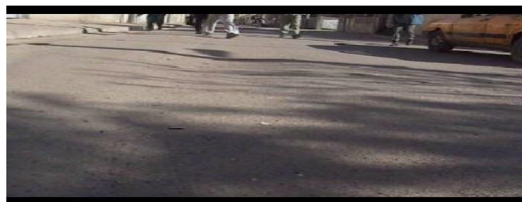
Fig (10) Rutting at AL- AL-Huriya City
