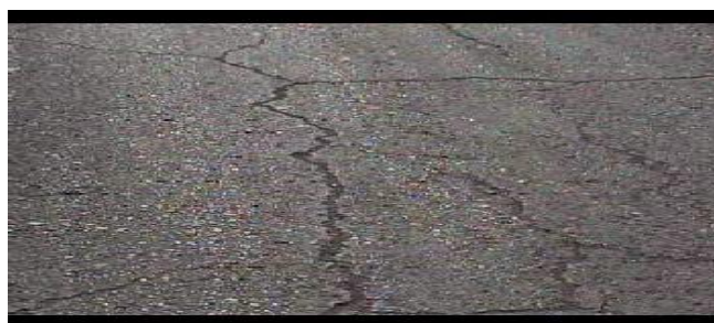
Fig (5) Block Crack at Al- Huriya City
