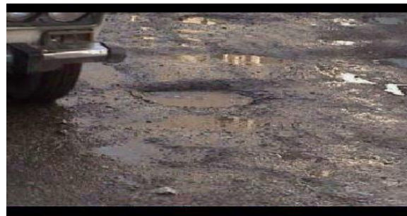
Fig (9) Pavement Potholes at AL-Huriya city
