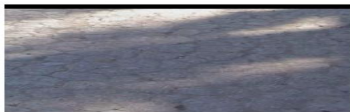
Fig (2) Alligator crack at AL- Huirya City
