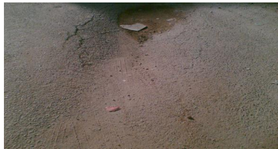
Fig (4) High Severity Depression at AL- Adel City
