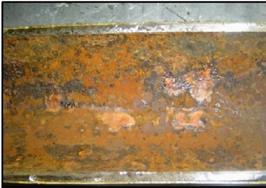
Figure 1. Internal corrosion of water injection pipeline.
