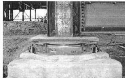
SF Airport Terminal Installed Bearing
