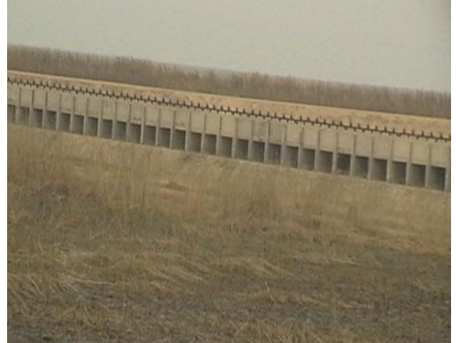
Figure 1. Hydraulic structures in Iranian dike at the coordinate in UTM (N=3474521.24891m, E =755381.586716 m), during 5-12-2012.
