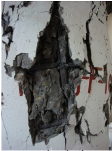
Plate 4 Spiral rupture occurs before complete spalling of concrete cover (HSC-F-100)
