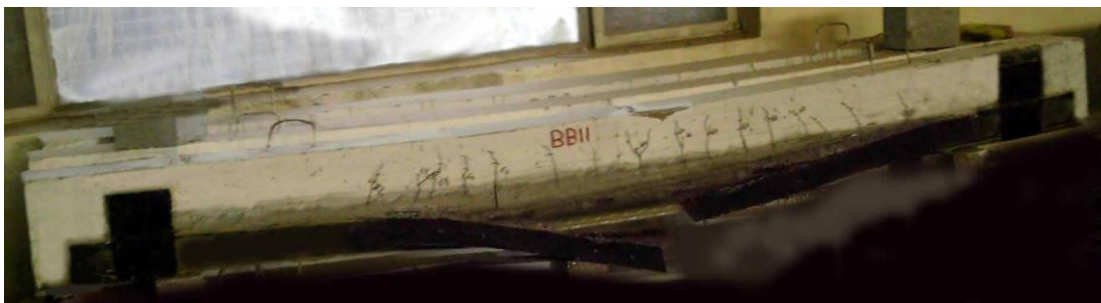
Figure 13 Crack pattern for beam BB11- strengthened beam (at sides of beam)
