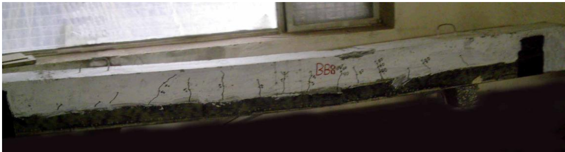
Figure 19 Crack pattern for beam BB8- (beam repaired by CFRP in side faces)
