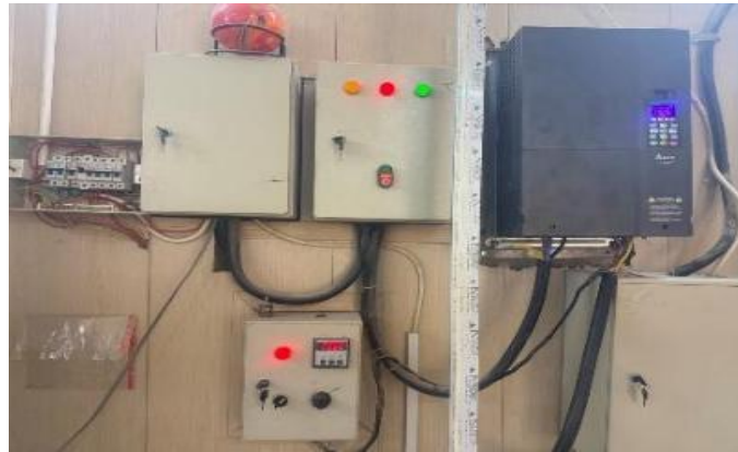
Figure 4. Electrical control panel and Delta C2000+ Variable Frequency Drive.
