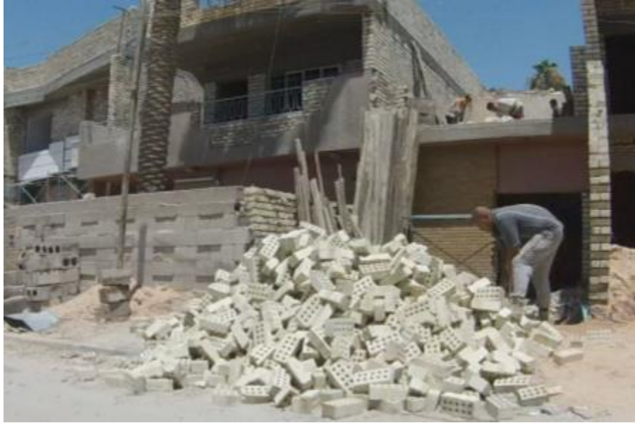
Figure 9. Workers without hard hats, gloves or any other personal protection equipment.
