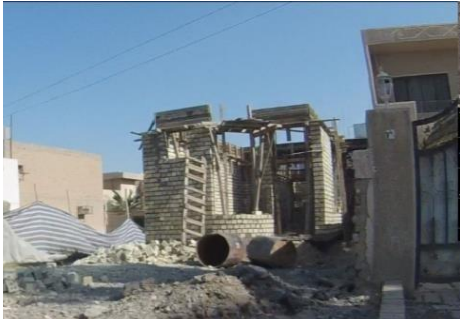
Figure 8. Non secured site, no warranty signs and potential falling objects.
