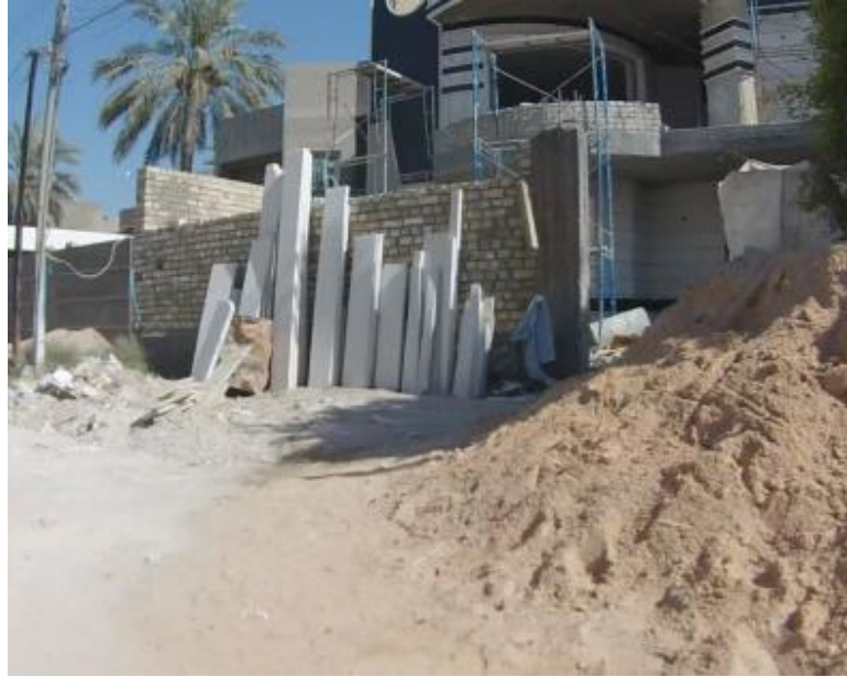
Figure 7. Non secure site with large heavy marble boards and unattended scaffold.
