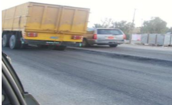
Figure 1. A Plate shows Rutting Occurring in Pavements.
