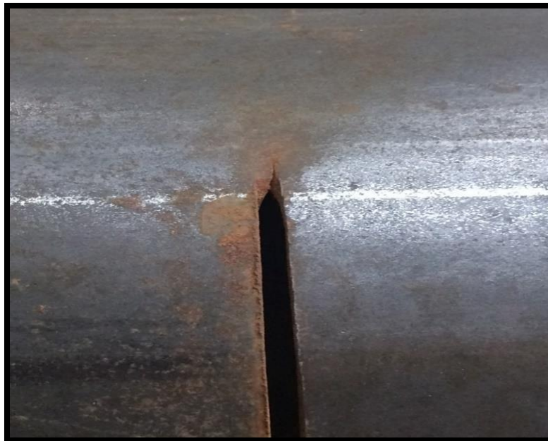
Figure 6. Close up photo showing the crack and crack growth.
