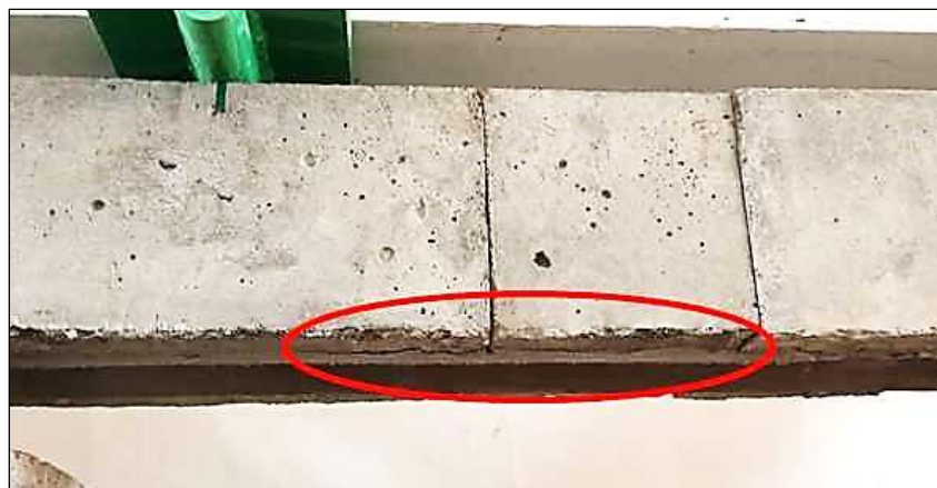
Figure 14. Partial debonding of EBR-CFRP in beam SB5-CFRP-950-GS-NA-2.0.
