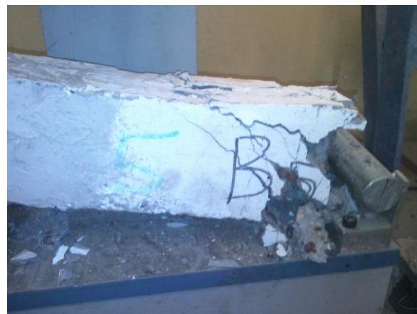
Figure 16. Failure of B5 after repair.
