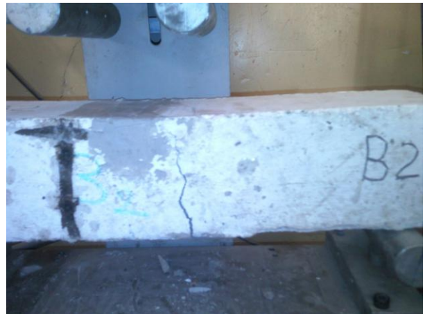
Figure 10. Failure of beam B2 after repair.
